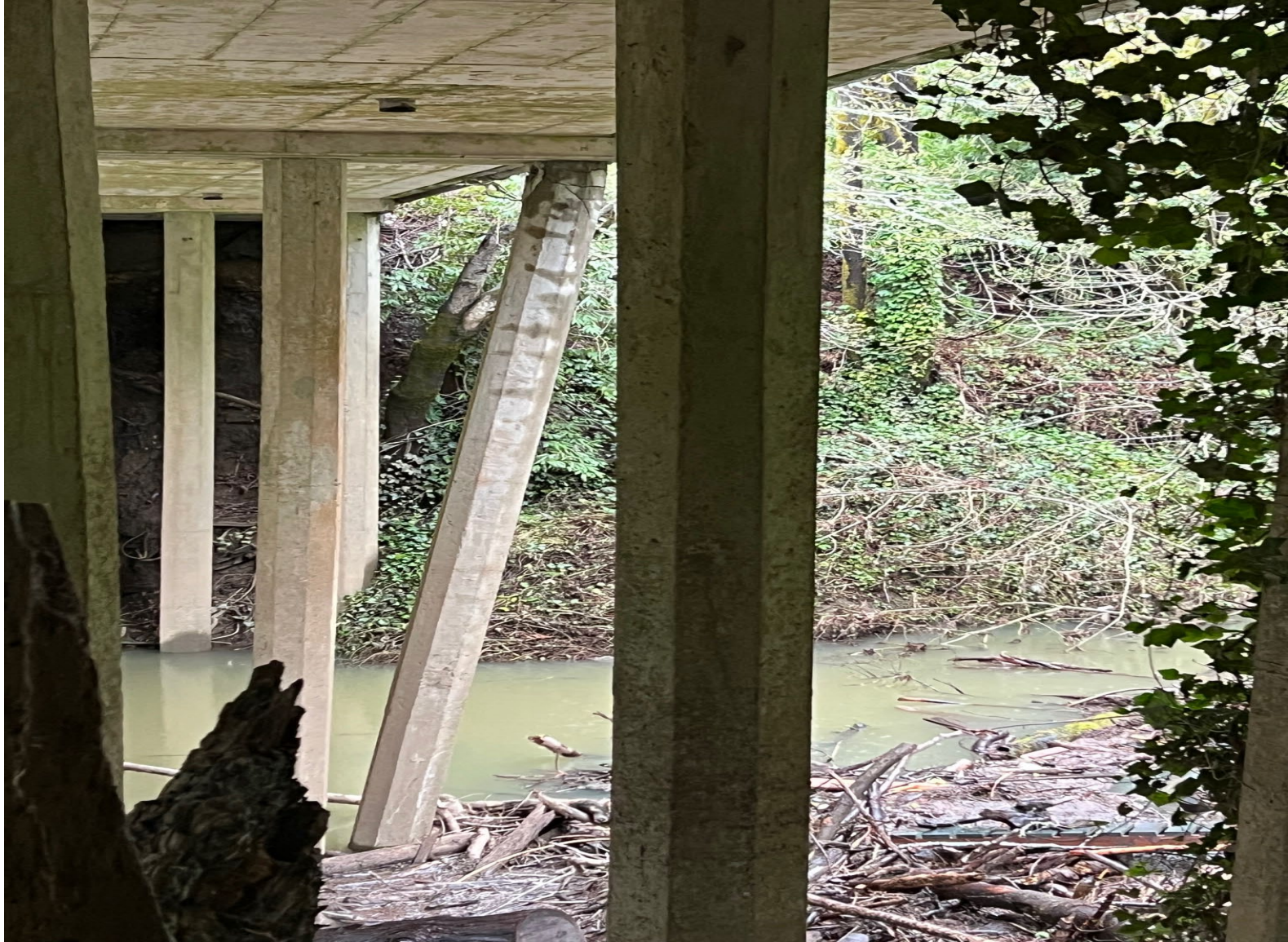
Damage Dutch Bill Creek Bridge Monte Rio, CA
